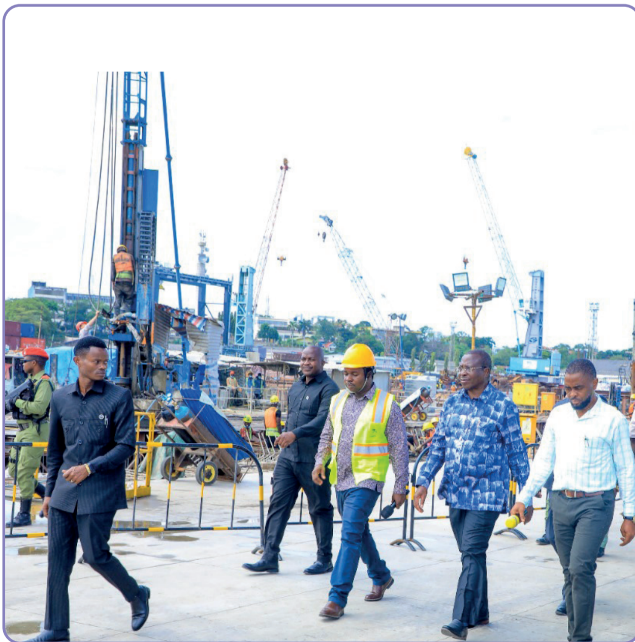
Vice President Dr. Philip Mpango (second – right) inspects Tanga Port improvement works, November 20, 2022 (Photo by Vice President's office ( www.vpo.go.tz ))
